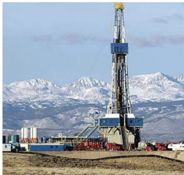
A Drilling rig drills for natural gas just west of the Wind River Range in the Wyoming Rockies (Photo credit: Wikipedia)
