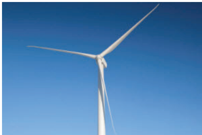
Tracking turbines: When Broken Bow 2 is completed, Sempra U.S. Gas & Power will have joint-venture projects totaling more than 1,000 megawatts (MW) of wind generating capacity.
