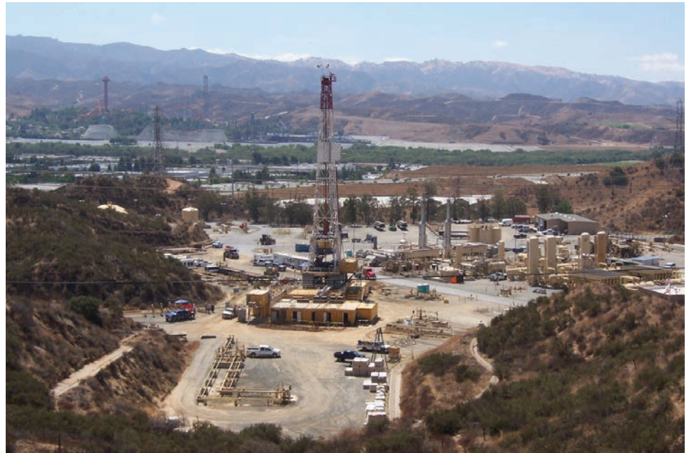
Ensign Rig No. 587 on site at Southern California Gas Company's Honor Rancho Gas Storage Field in Los Angeles County, CA.
